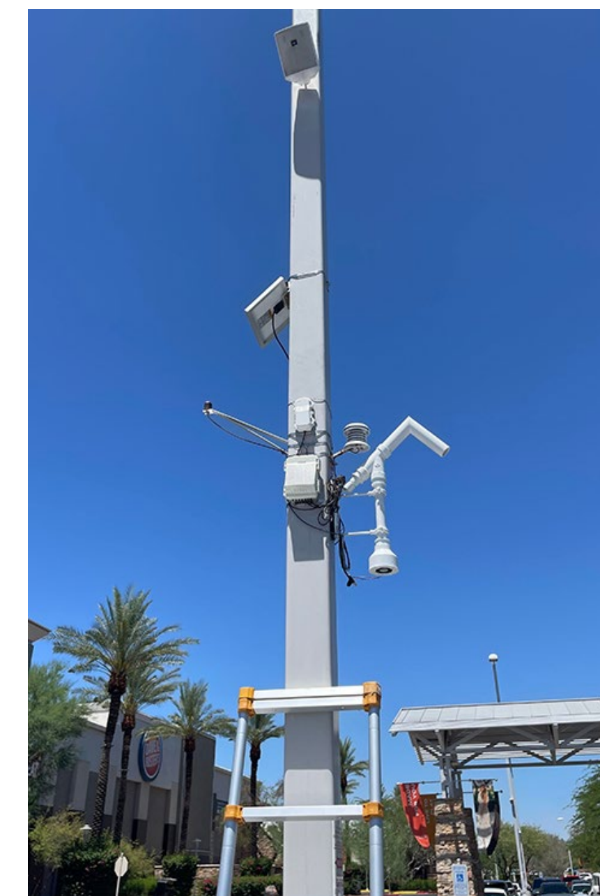
Fig. 2: left: Aspirated sensor assembly (double-walled configuration); right: the picture of installed aspirated and non aspirated sensors at 3m height
